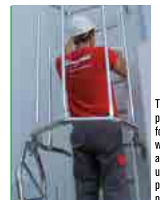
The trapdoor provides a safety exit for operators while preventing access to unauthorized persons: passive safety.
